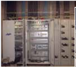
Control Panel and Motor Control Center
